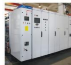
超级电容储能装置 Ultra capacitor energy storage device
